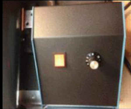
MOTOR CONTROL BOX
